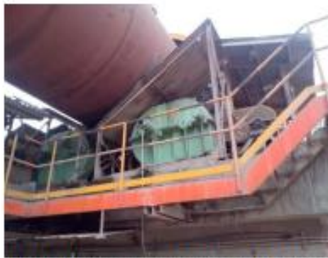
Reductores mando principal horno base 2
